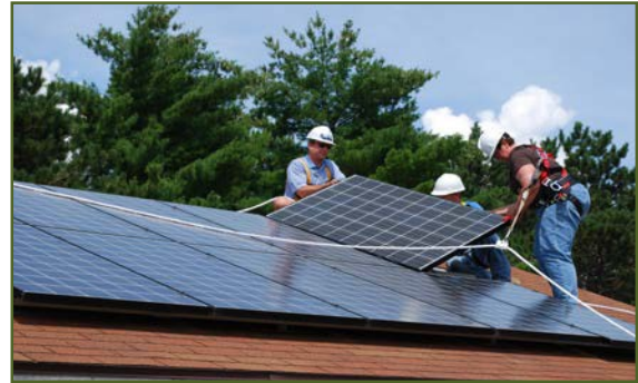
Rooftop Solar, MREA
