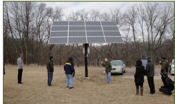
Ground Mount System, CERTs
