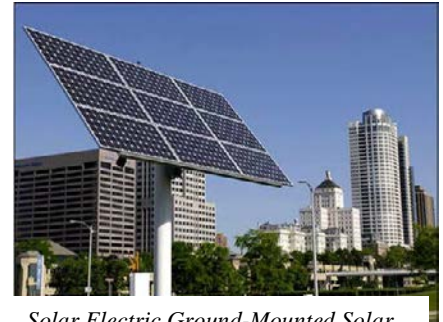
Solar Electric Ground-Mounted Solar Array at Discovery World
